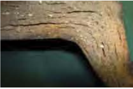
100+-year-old pipe wall with laminations created when the pipe was manufactured
